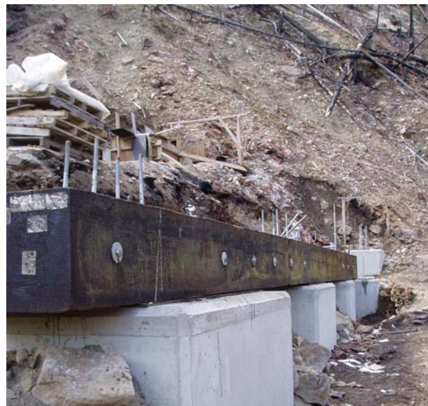
Figures 22, 23, 24, 25. Trestle 4 required the installation of over 150-25' long micropiles – all placed using portable equipment
