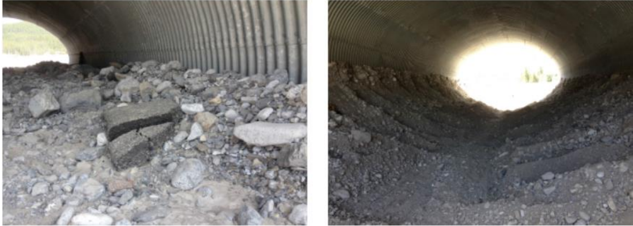
Figure 18 - Debris Accumulation Inside Conduit from Event (Before and After)
