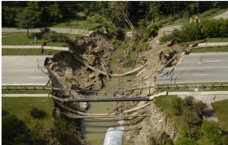
Figure 4 - Structure and Soil Damage
