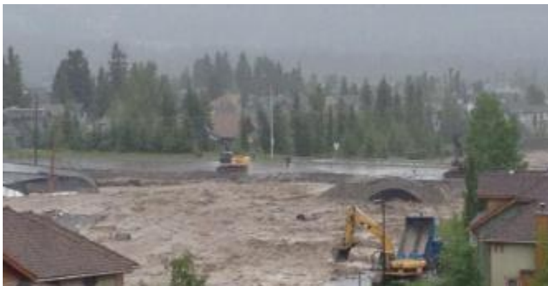
Figure 17 - Cougar Creek Washout During Extreme Hydraulic Event
