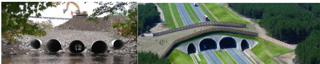
Figure 3 - Multiple Conduit Crossings
