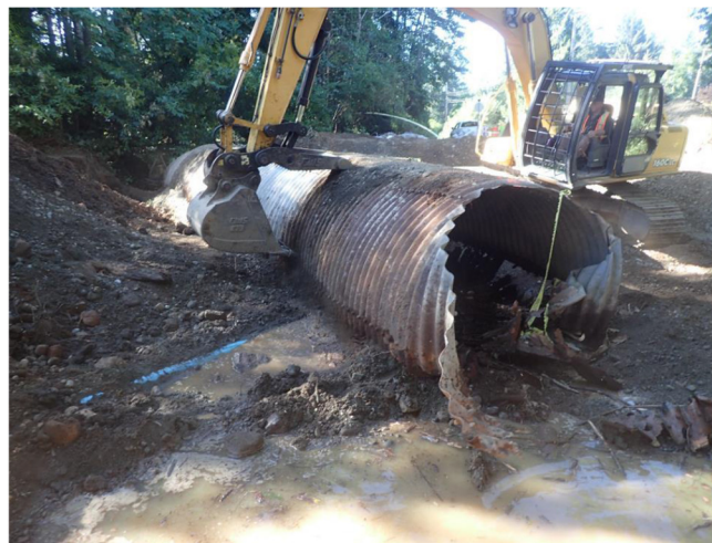
Figure 10: Structure at End of Service Life (photo courtesy of Sean Wong, BCMOTI)
