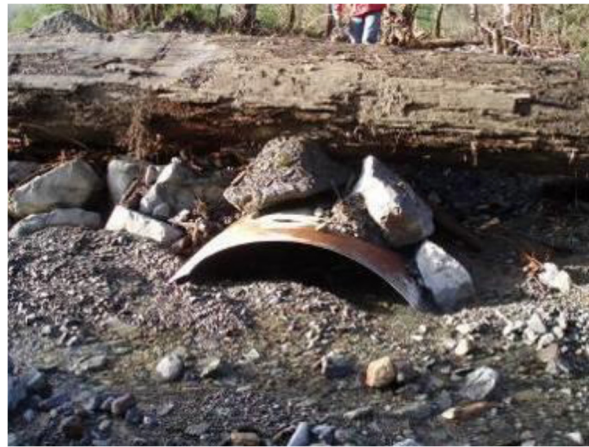
Figure 3: Blocked Culvert (photo courtesy of Sean Wong, BCMOTI)
