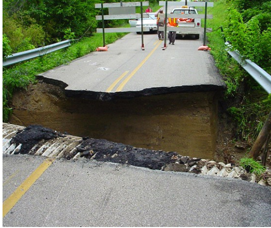
Figure 4: Scouring Washout Leading to Road Closure (Butler County Engineer's Office, 2001)
