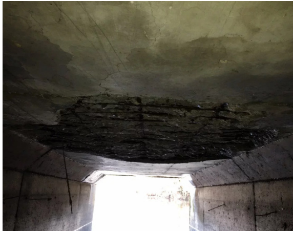
Figure 5: Spalling Resulting in Four Month Closure (Cline, 2015)
