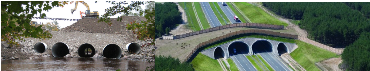
Figure 1 - Multiple Conduit Crossings
