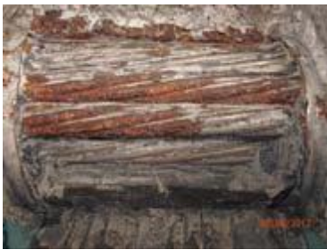
Figure 7. Corrosion of post-tension tendons in soft grout (Florida Department of Transportation 2013)
