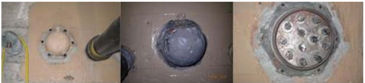
Figure 19. From Left to Right: Before removal of anchor cap, view of grout at anchorage after anchor cap was removed, and exposed anchor plate and strand ends after removal of grout
