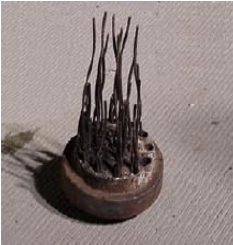
Figure 2. Failed tendon due to corrosion near anchor plate. (Florida Department of Transportation)
