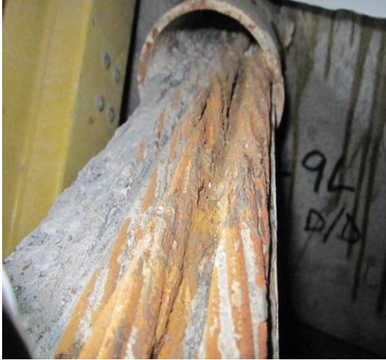
Figure 1. Corrosion evident in voids in a tendon duct near anchorage. (Florida Department of Transportation)
