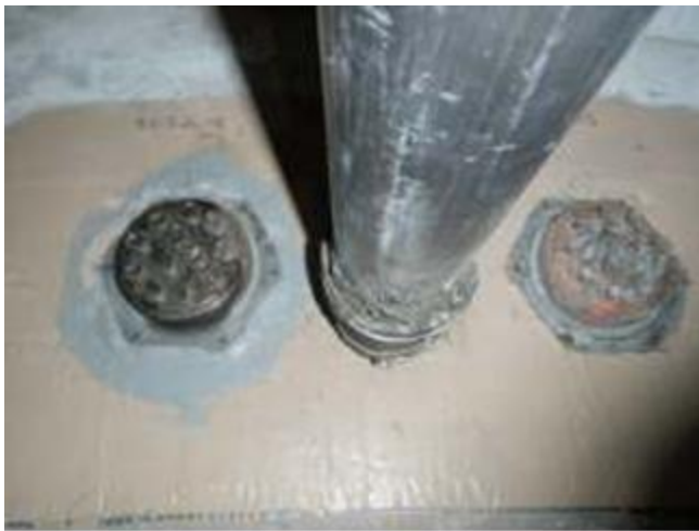
Figure 22. Post-Tension Impregnation Material present at far end of tendon on left. No impregnation material present on adjacent tendon (right).
