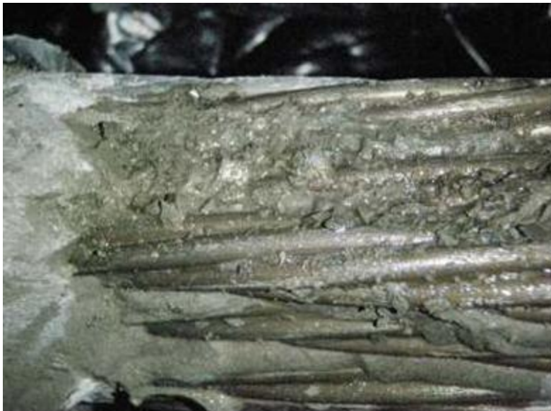
Figure 25. Post-Tension Impregnation material clearly visible in the strands as well as in the surrounding grout
