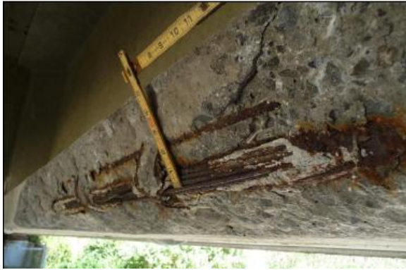
Figure 5. Voids between wires, high water cement ratio grout and presence of chlorides does not provide adequate corrosion protection to the PT tendon.
