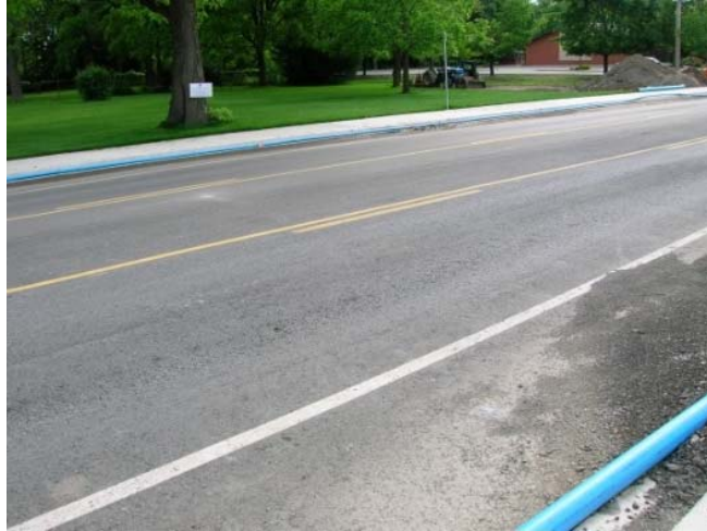
Figure 7. Raveling of new binder course mix that incorporated very high content of RAP.
