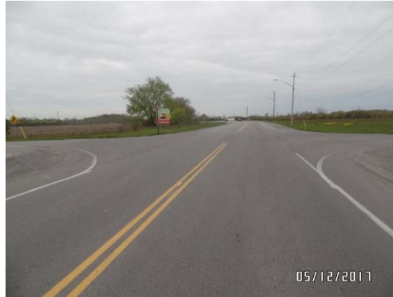
Figure 12. Excellent current condition of asphalt pavement placed in the Region of Niagara in 2016.
