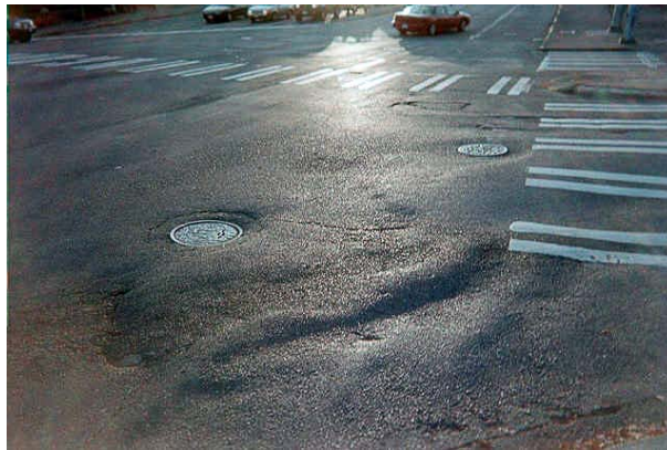
Figure 1. Frost heaving deformation at an intersection in a vicinity of a manhole.
