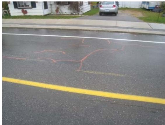
Figure 9. Cracking of new binder course that contained high percentage of RAS.
