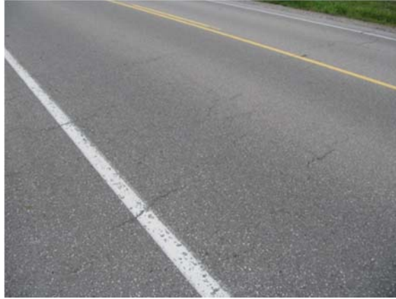
Figure 5. Check cracking on Moser Young Road in Region of Waterloo.
