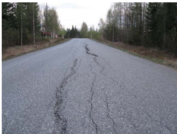
Figure 2. Severe cracking on a rural pavement due to frost heaving.
