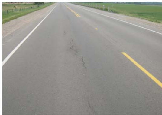
Figure 3. Midlane cracking of a 6 months old pavement on Bleams Road in Region of Waterloo.
