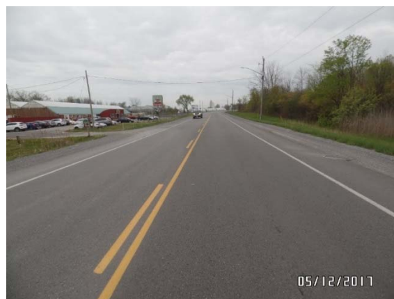
Figure 11. Excellent current condition of asphalt pavement placed in the Region of Niagara in 2016.
