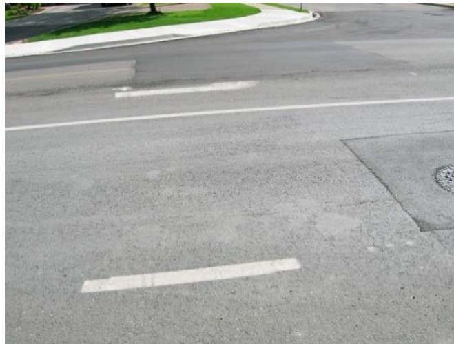
Figure 8. Raveling and cracking of new binder course that incorporated very high content of RAP.
