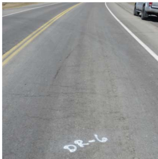
Figure 4. Premature pavement cracking on Region of Niagara Regional Road 25 Doan's Ridge Road.
