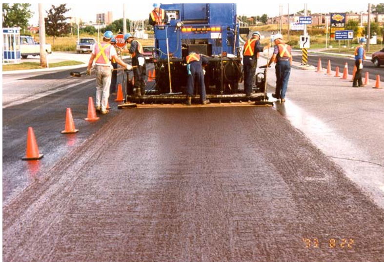
Figure 3 – Rut filling with microsurfacing lower lift on Thickson Road in Whitby, Ontario in 1993.
