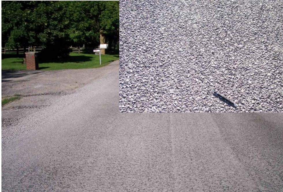
Figure 1 – Chip seal applied on Coates Road in Oshawa, Ontario in 2004. The close-up shows the surface treatment.
