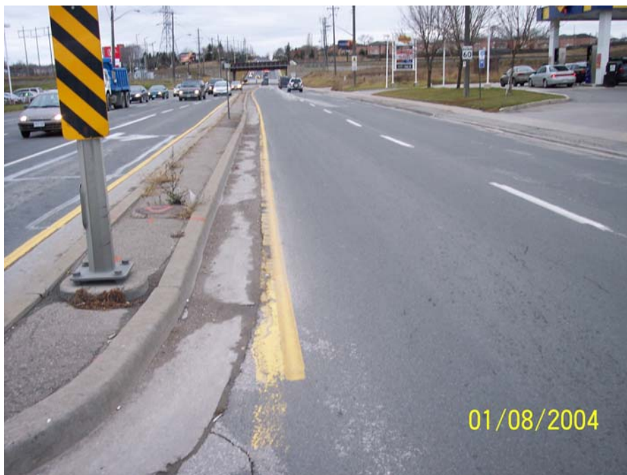
Figure 5 – Condition of microsurfacing on Thickson Road in Whitby, Ontario in 2004.
