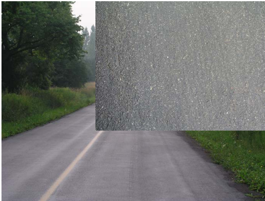
Figure 2 – Cape seal applied on Hall's Road in Whitby, Ontario in 2003. The close-up shows the surface texture.
