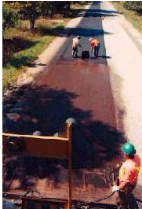
Figure 6 – Application of Metro-Mat (TM) on Wellington County Road 42 about 20 km west of the City of Brampton, Ontario
