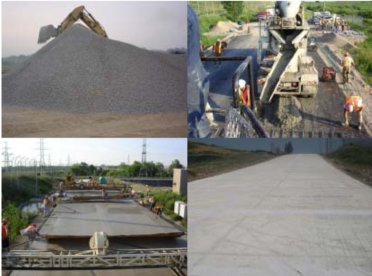
Figure 3 Clockwise from Top Left: RCA Stockpile, Concrete Pavement Placement, Finished Concrete Pavement Surface, Finished Concrete Pavement
