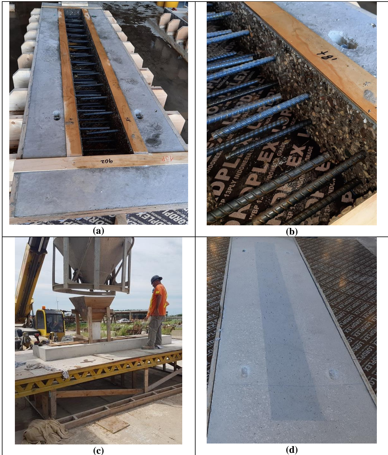
Figure 2: UHPFRC Mock-up (a) After Casting the Normal Concrete Part, (b) Exposed Aggregate Finish of the Normal Concrete, (c) Casting the UHPFRC Joint and (d) After Curing and Grinding the UHPFRC Joint
