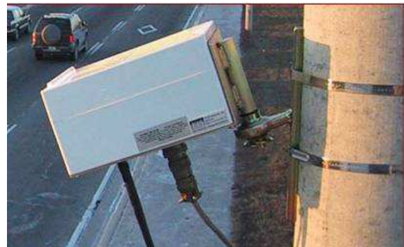
Figure 3-2 Side Fired Vehicle Detector
