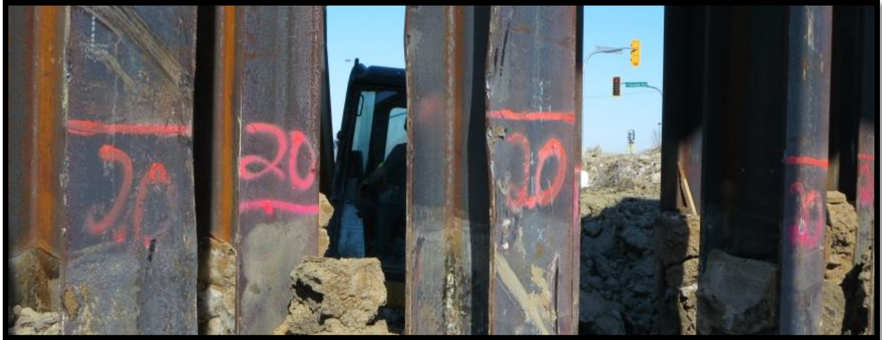
FIGURE 9: DAMAGED EAST ABUTMENT PILES
