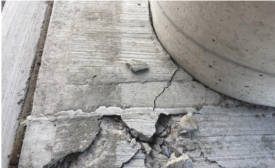
Photograph 7 – Not Providing Isolation Joint
