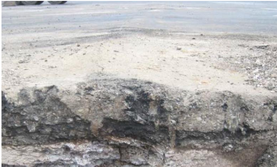
Photograph 9 – ASR-induced swelling of concrete under asphalt overlay.
