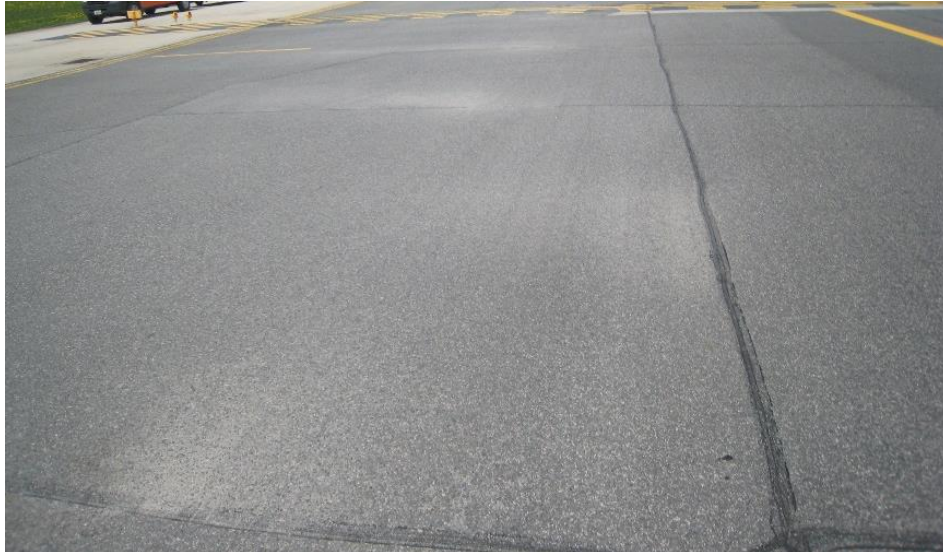
Photograph 6 – Pumping of fines through longitudinal and transverse joints
