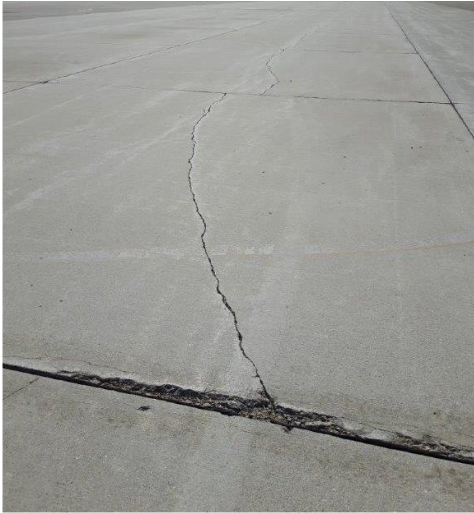
Photograph 11 – Full depth longitudinal crack due to the presence of a utility trench under concrete slabs
