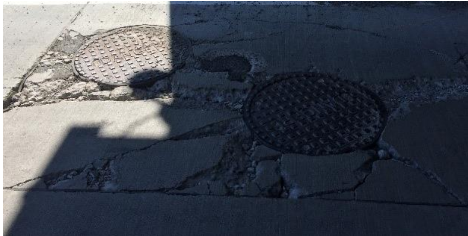
Photograph 8 – Concrete slab shattered into pieces due to failure to adhere to good design and construction fundamentals
