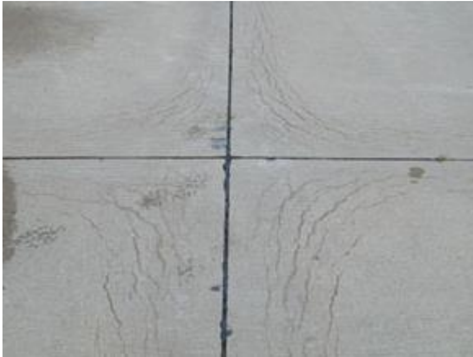
Photograph 10 – D-cracking of concrete pavement
