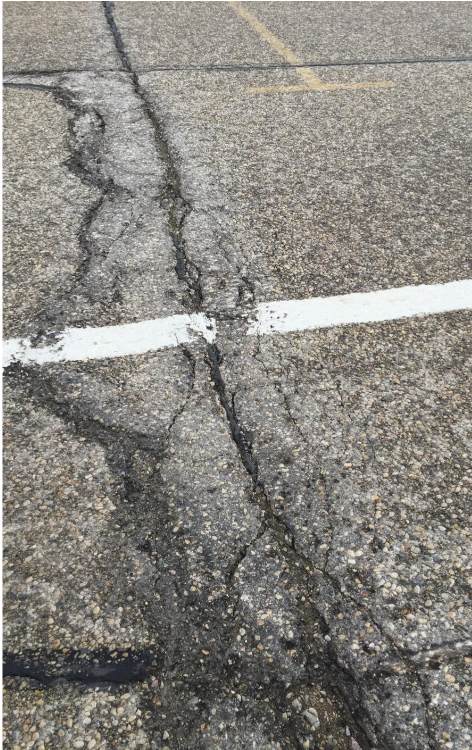
Photograph 5 – Frost heaving of concrete slabs unsuccessfully repaved with asphalt overlay
