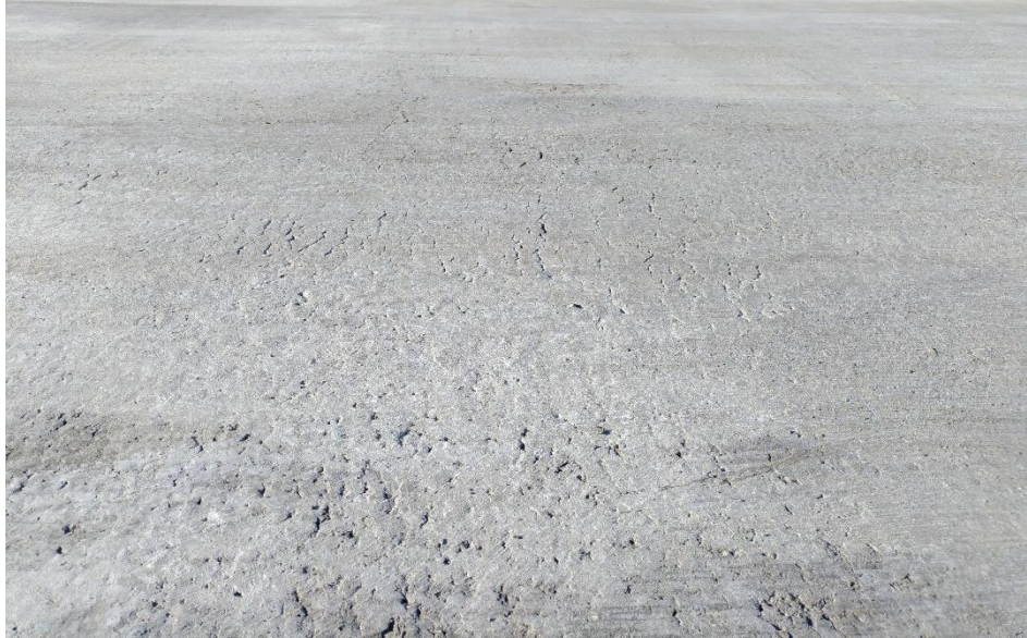
Photograph 14 - Poor concrete consolidation and finishing work
