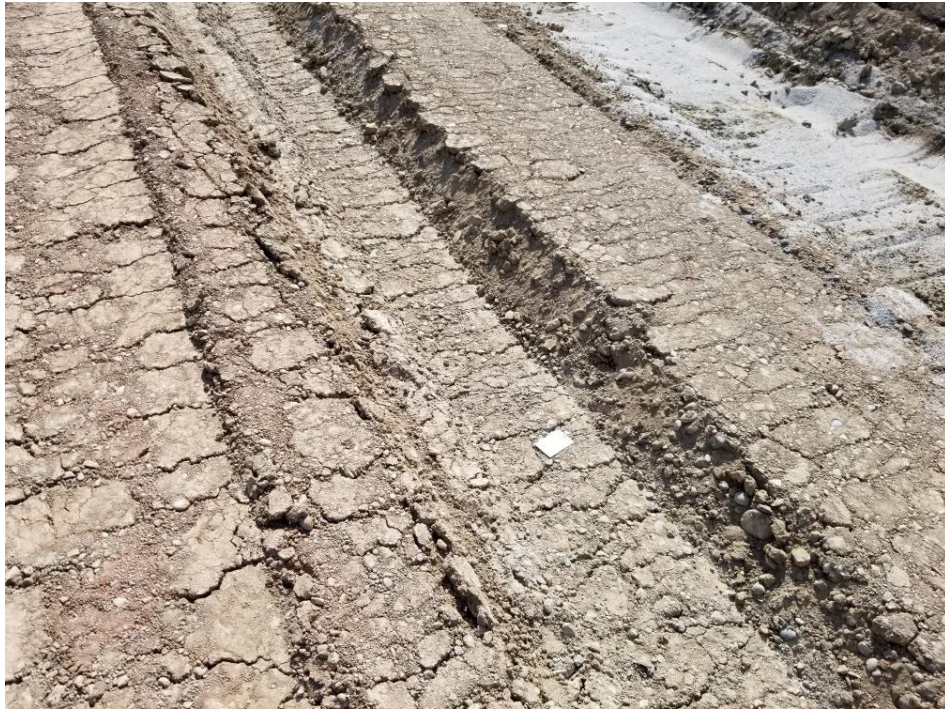
Photograph 4 – Soft subgrade soil that failed proofrolling. Further work is needed prior to placing base course.
