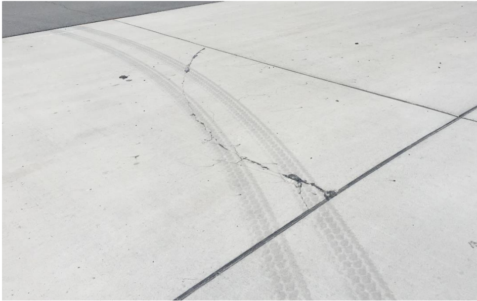
Photograph 12 – Severe corner break due to inconsistent support
