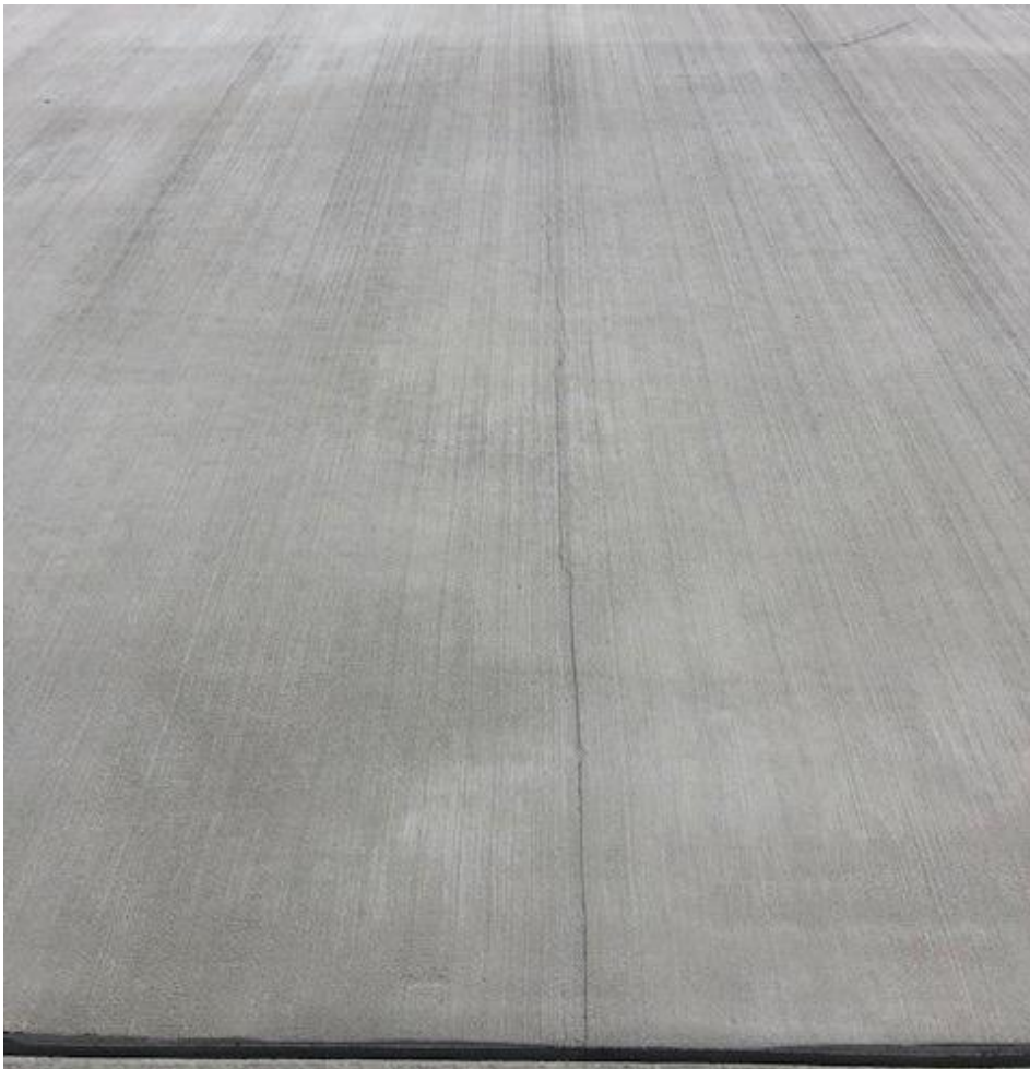
Photograph 13 - Full depth longitudinal crack due to inconsistent support
