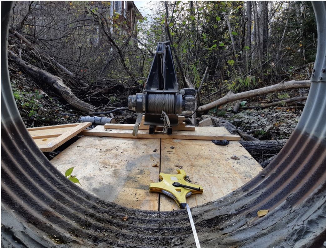
Figure VII – Winch at Site NE12
