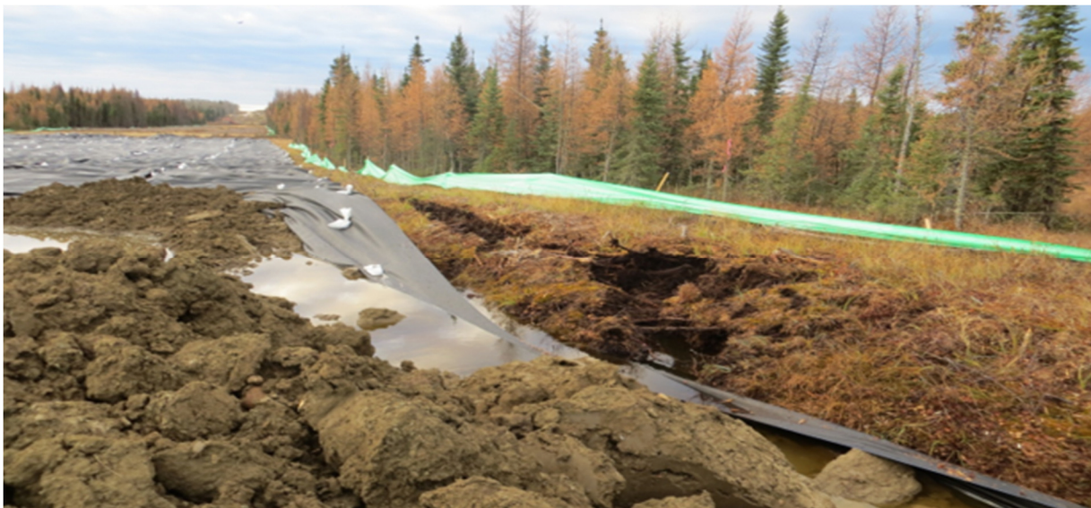
Photo 5.5: shear failure within muskeg zone during placement of initial fill lift
