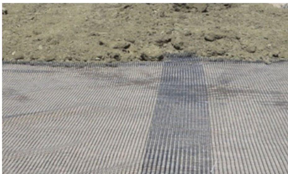
Photo 3.1: Placement of biaxial geogrid within lower level subbase/subgrade construction. Rolls of geogrid product are overlapped and spread out evenly across the grade and then uniform layers of suitable fill materials are placed and compacted above to create a stable surface for further grade construction.
