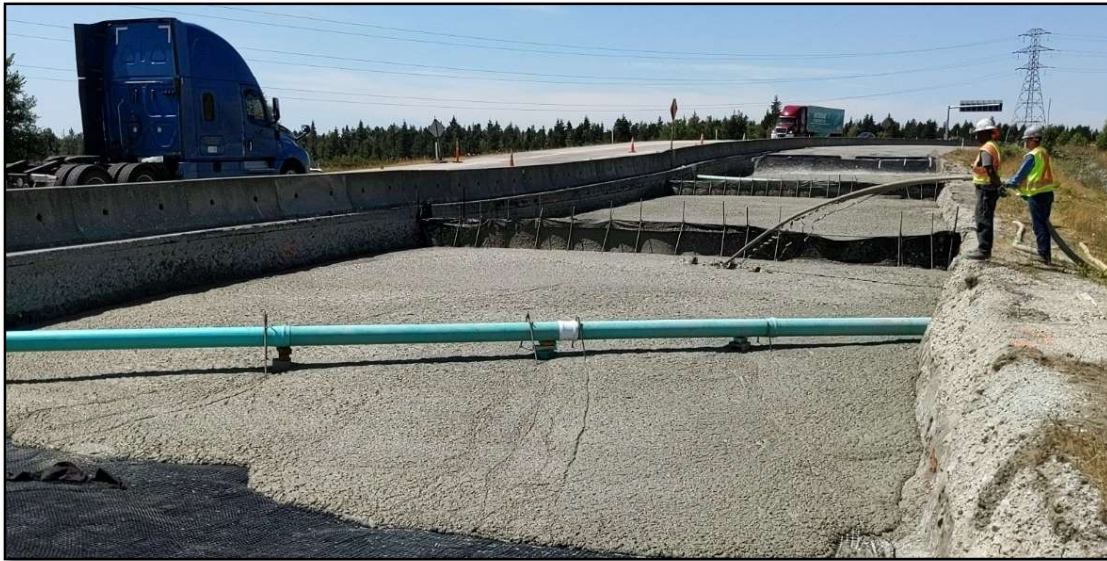
Figure 4: Construction of Light-weight Cellular Concrete (LCC) fill being placed in terraced steps. Partitions, made of geotextile and rebar, were utilized between the steps of different elevations and/or depths of LCC fill.
