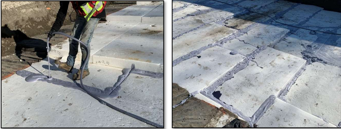
Figures 6 & 7: Application of high-density expanding polyurethane closed-cell foam via injection to fill the voids between the EPS blocks.
