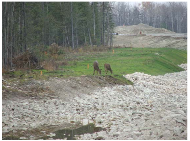
Figure 9 Construction Challenges: Keeping up with the deer consuming all of the tasty fresh grass was a constant challenge. The deer removed all of the grass growth in this area in a couple of days.
