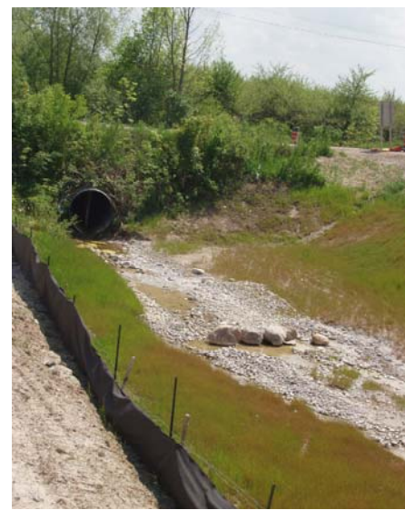
Figure 3 Nottawa Side Road with Watercourse Channel Installed: The watercourse features and side slopes were installed and let stabilize prior to culvert removal.
