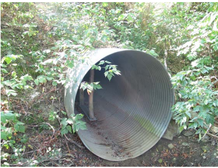
Figure 2 Old Steel Culvert Under Nottawa Side Road: This culvert was removed and the side road cull de sac pulled back to provide room to create a naturalized valley and watercourse with natural channel design features. This is located at the easterly side of the new highway.
