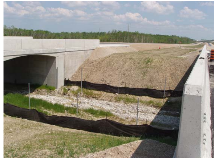
Figure 7 Open Area Between Wildlife Structures Allows Deer Good Visibility to Identify Predators and Safely Use the Passage
