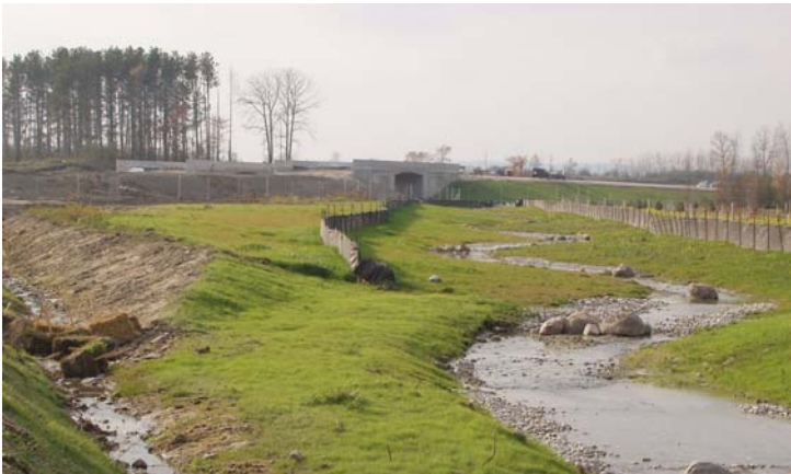
Figure 6 View of Nottawa Side Road Watercourse with Completed Channel: Water now flows freely from the abandoned orchards, downstream through the deer/wildlife crossing. This watercourse is now utilized by rainbow trout. It was formerly home to only small baitfish such as minnows. Deer and other wildlife use the grassy areas to cross.
