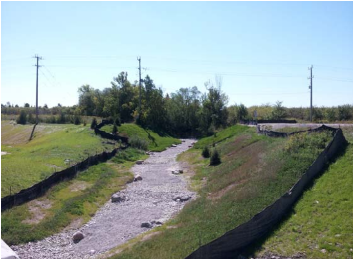
Figure 4 Nottawa Side Road Valley and Water Course Completed "In the Dry": The old steel culvert has been removed, the channel substrate installed and the new valley opened to the abandoned orchards.
