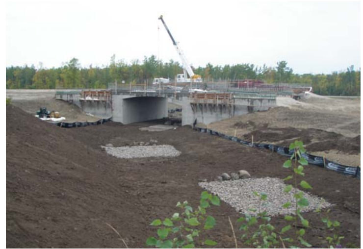
Figure 5 Construction of the Deer/Wildlife Crossing Structure: These two structures allow wildlife to pass under the new highway. The rectangles of river stone and the larger boulders are the initial stages of the installation of the naturalized channel for the small watercourse at Nottawa side Road.
