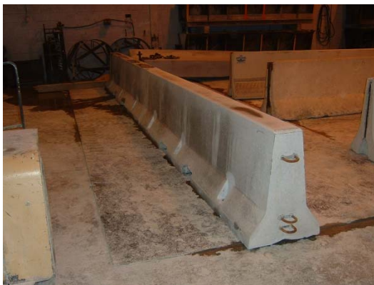
Figure 1: Type M Temporary Concrete Barrier (MTO File Photo)
