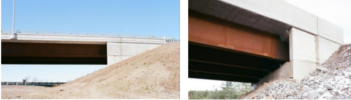
Fig. 4. Typical semi-integral abutments of new steel girder bridges. Note the leakage from the joint in the barrier wall onto the wingwalls.
