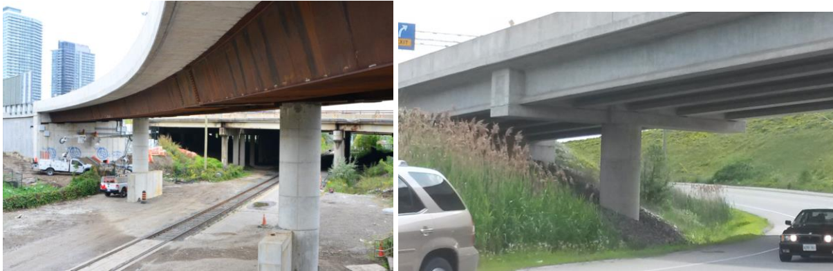
Fig. 11: Curved composite steel tub girder bridge, and straight precast concrete girder bridge supported on integral pier without bearings
