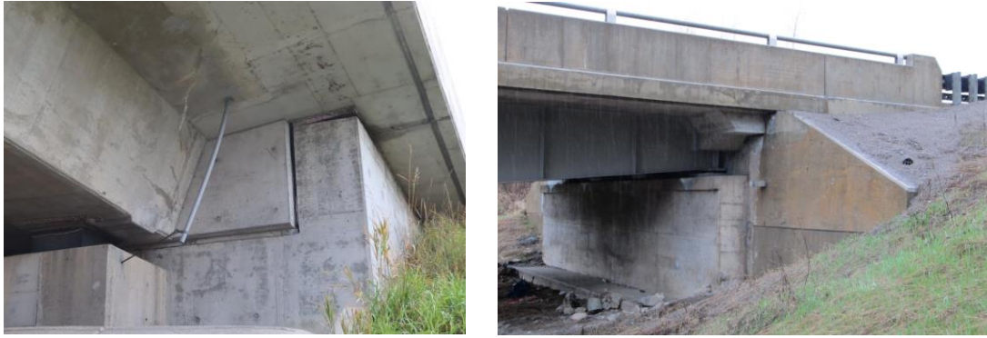
Fig. 7: Semi-integral abutment details with the barrier continuous from the deck onto the approach slab (overhanging the wingwall in the first image, cast on grade in the second)
