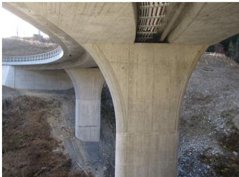
Fig. 12: Spinatobelbrücke, example of a cast-in-place post-tensioned bridge on integral abutments (flexible walls) in Malix, Switzerland (image courtesy of Tiefbauamt Graubünden)
