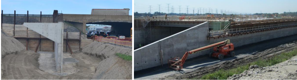
Fig. 18: Photos of construction of IABs on shallow foundations where a solid wall provides flexibility above a spread footing. On the example in the right, the wall is partially backfilled prior to casting the frame corner connection between the deck and walls
