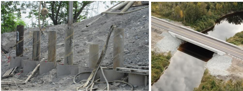
Fig. 15: HSS 356x16 piles supporting the Flagg Road Underpass over Hwy 401 during installation, and the Hwy 101 Ivanhoe River Bridge, supported on three 610 mm diameter concrete filled steel tube piles
