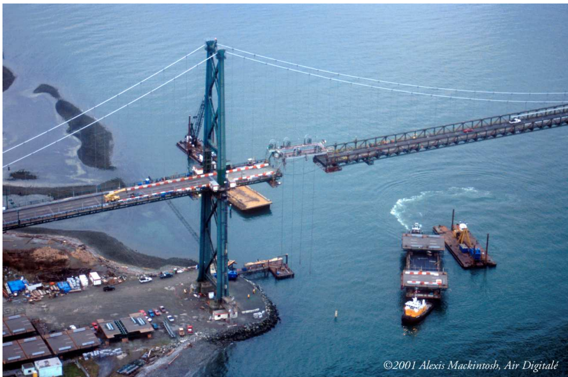
Figure 4: Temporary gap in Lions' Gate Bridge as a segment is being replaced
