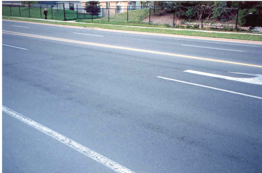
4. Example of generally poor overall quality (poor appearance) with poor transverse and longitudinal joints, mat texture variability, raveling and some low severity reflection cracking.
