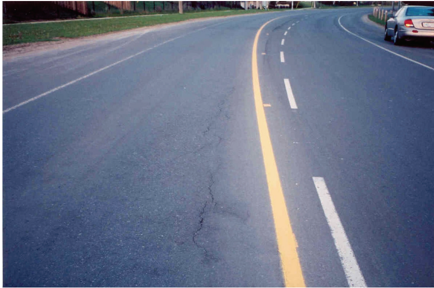
5. Example of generally poor overall quality (poor appearance) with poor transverse and longitudinal joints, texture variability and, particularly, medium to high severity longitudinal reflective cracking.
