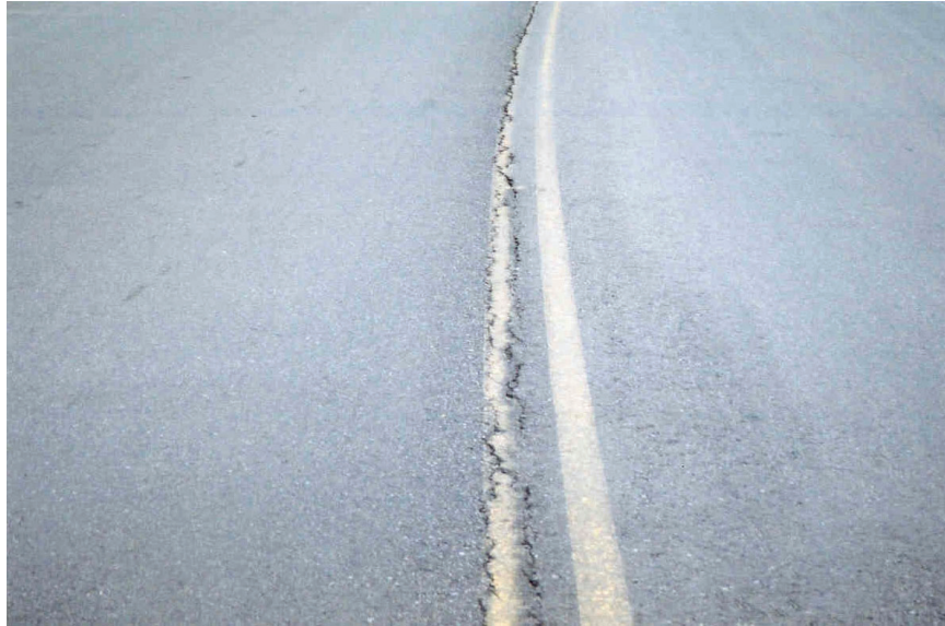
3. Example (close-up) of an open and medium severity cracking longitudinal joint (progressive deterioration) due to poor construction practices ('cold' weather paving, poor compaction of joint area and no joint tacking for instance).
