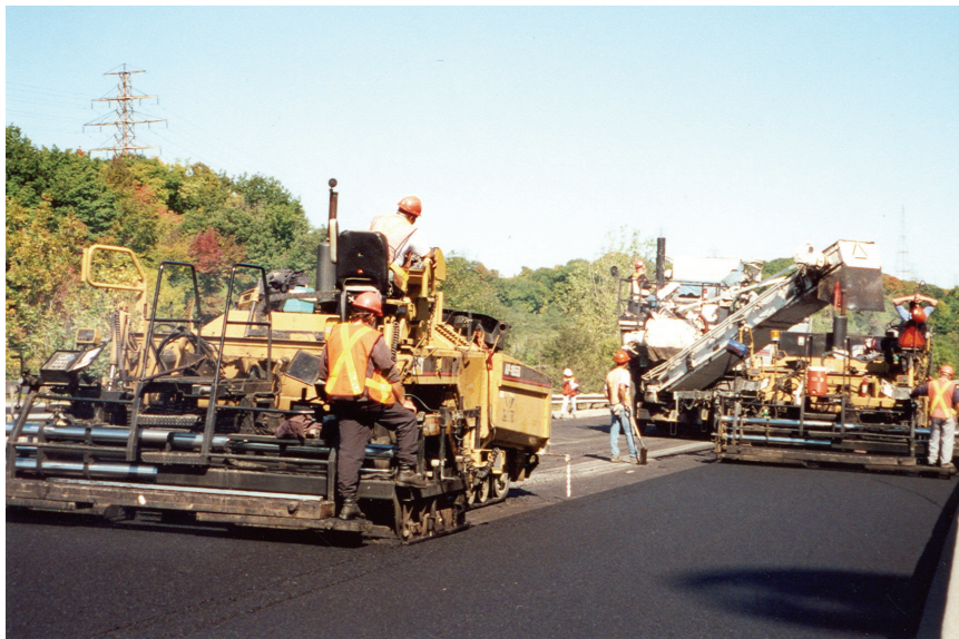
6. Placing stone mastic asphalt (SMA) surface course as long-life asphalt pavement with two pavers in echelon and a material transfer vehicle (MTV).
