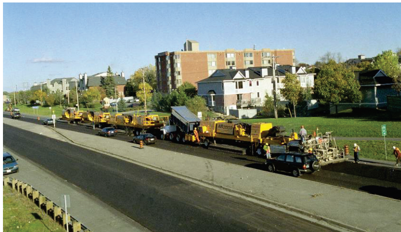
Photograph C131 - Current HIR Remixing train rehabilitating a municipal roadway in a single pass
