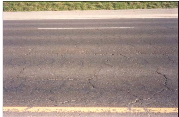
Photograph C19-1 showing map cracking distress caused by steel slag aggregate
