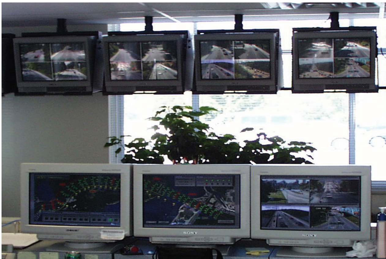
Figure 12 - RLS Central Control System, Vancouver, B.C.
