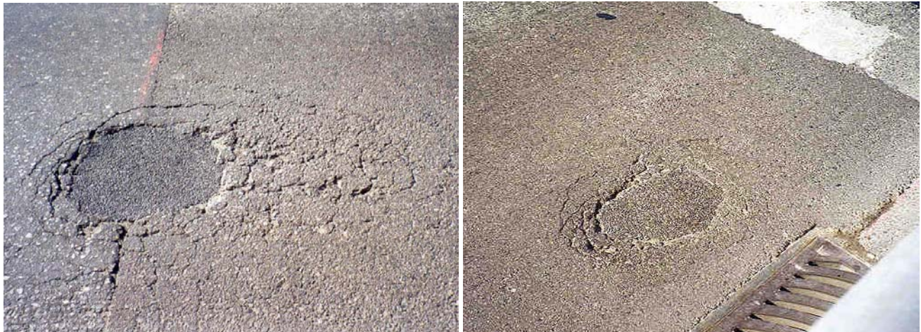
16. Close-up of Typical Asphalt Concrete Patch, Cracking, Blistering and Potholing of the Asphalt Concrete for the Oak Street Deck Rehabilitation (Photograph 15) Due to Performance Problems with the Sheet Membrane Waterproofing System, Vancouver, 1998.
