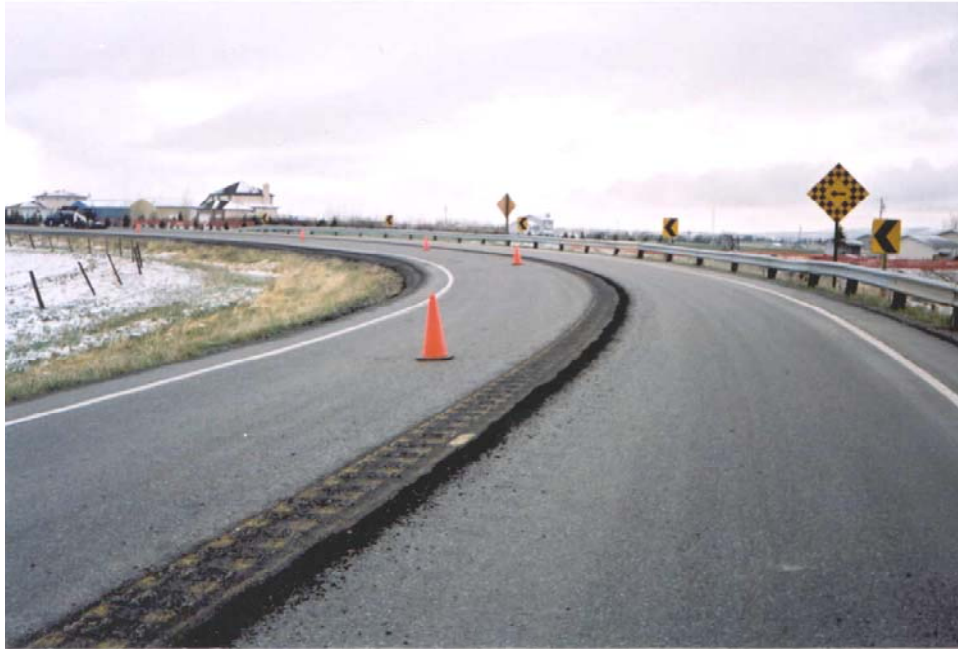
Figure 2: An example of milled CLRS in Alberta (Photo: Dr. John Morrall; Equipment Courtesy: All West Bobcat Services)
