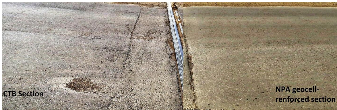
Figure 3 CTB section on left and NPA Geocell-reinforced on right side of rail track one year after construction, summer of 2013. (reproduced from Pokharel et al. 2017)
