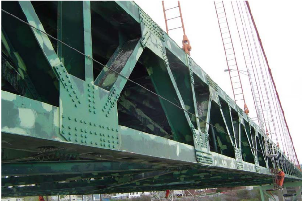
Figure 4. Suspension Bridge Longitudinal Stiffening Truss prior to Addition of Maintenance Access Walkways in 2007
