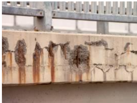
Figure 4 – Impact of de-icing agents on road network infrastructures
