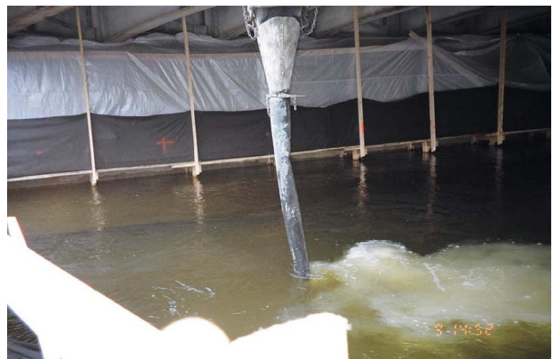
Figure 9: Slinger with a pipe trunk system installing the gravel liner underneath the structure. Photo by Jewel Eng.
