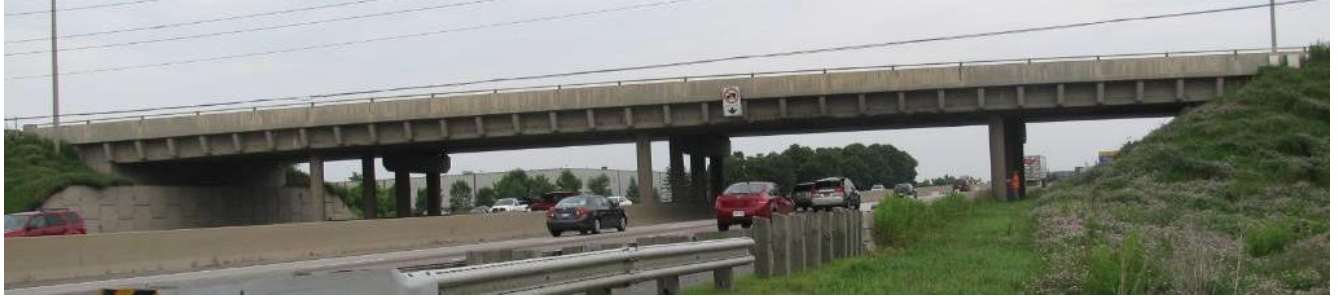
Fig. 7. Franklin Blvd Underpass over Hwy 401, the first integral abutment bridge in Ontario built 1962, shown with 1992 widening with cantilever brackets in front and twinning behind
