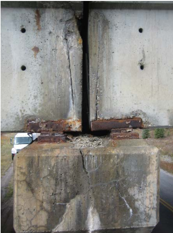
Figure 8) Cracked pier cap with severe corrosion of steel rocker bearings
