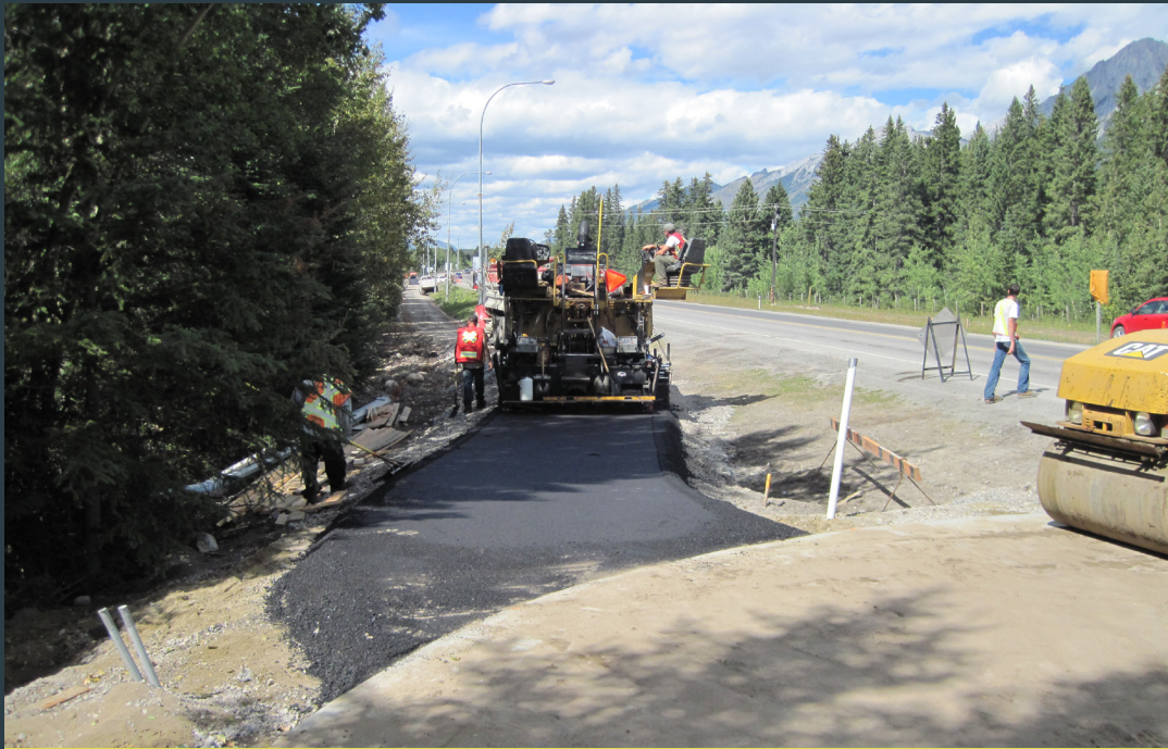
Workers paving up to the trailhead in Canmore, where the trail ties into the municipal trail network and the ROAM intercommunity transit system
