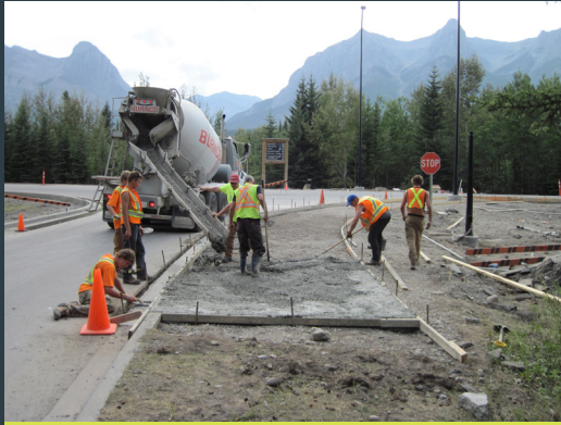
Installation of new concrete sidewalk to connect to parking lot expansion at the Travel Alberta Visitor Information Centre in Canmore
