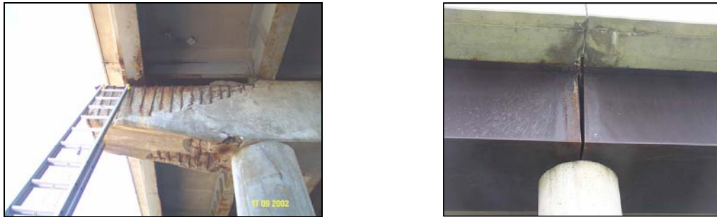
Figure 2: Typical Corrosion Damage Caused by Leaking Deck Joints
