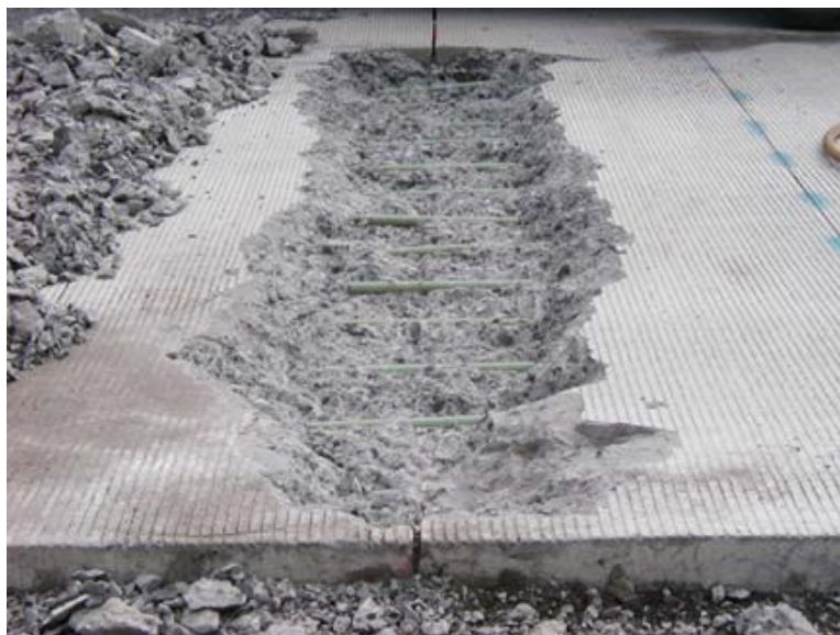
Figure 5: Chipped Out Transverse Joint with Dowel Bars Exposed
