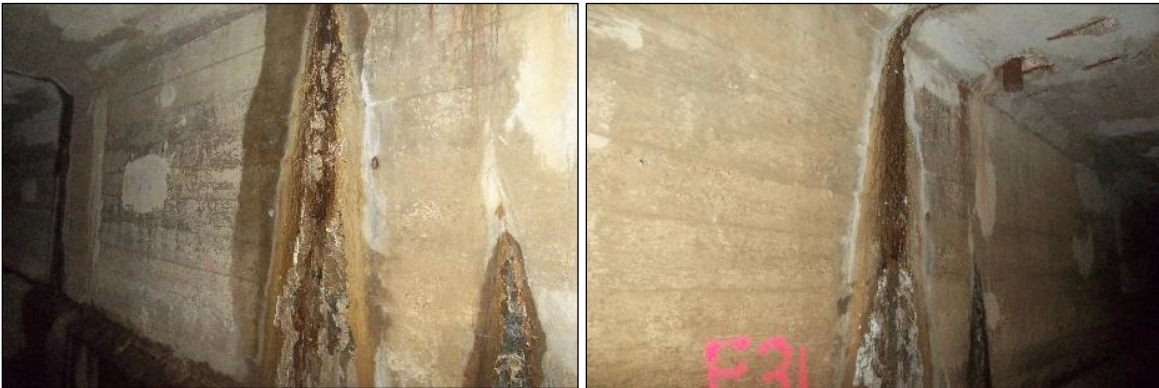
Figure 14 – Deterioration of Interior Walls in Box Culverts
