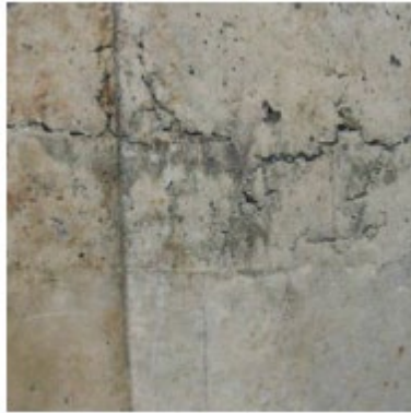
Figure 3: Typical Cement Cold Joint
