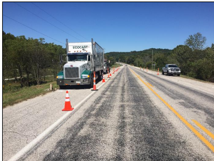
Figure 9 – SR 446 above Culvert needing Repair
