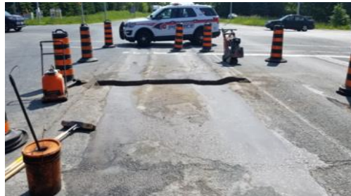
Figure 1: Rutting in Approach Intersection at Heavy Truck Traffic Road in York Region
