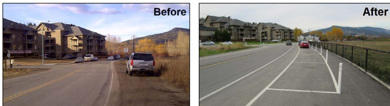
Bottom Wood Lake Road (Lake Country, BC): Photos show corridor improvements made in 2014, using a $53,000 contribution from the Road Improvement Program.
