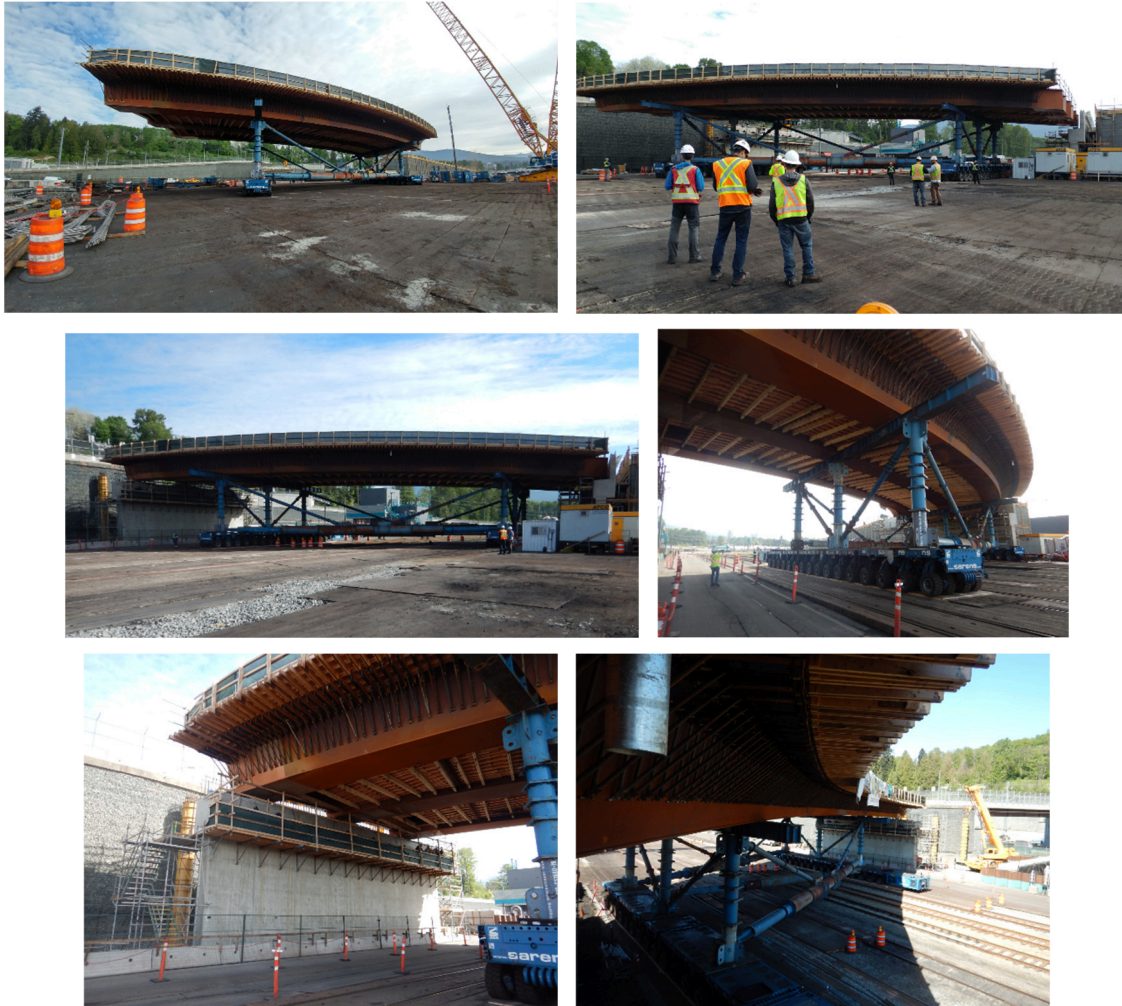
Figure 18: Girder erection completed with the use of Self-propelled modular transporters (SPMTs), Girders moved from staging area to final position above bearings
