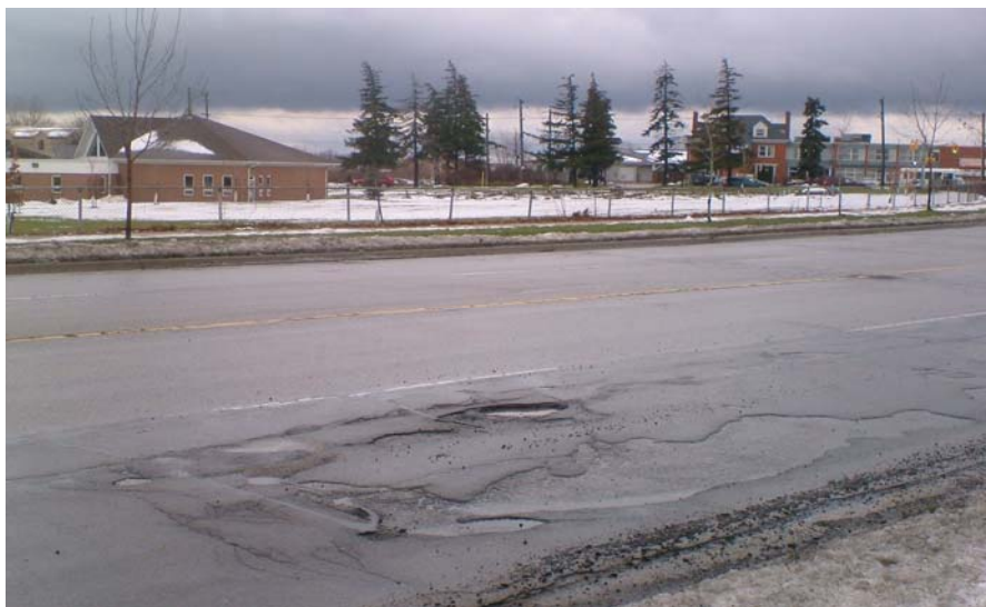
Fig.9, deteriorating pavement condition along many sections of Davenport Road
