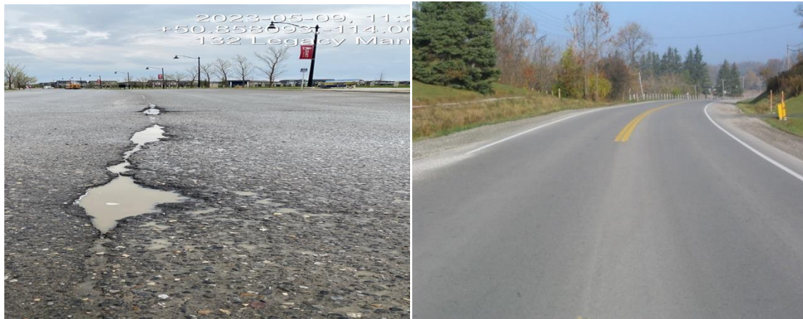
Figure 2 (a) Poorly Constructed; (b) Well constructed Longitudinal Joint [3]
