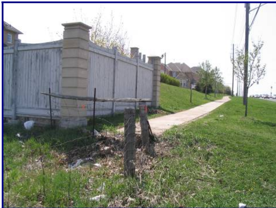
Figure 5 – Missing Links in the Existing Sidewalk System Were Identified (MMM Group Ltd.)
