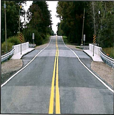
Photo 1: Geothermal Snow-Melt Bridge
