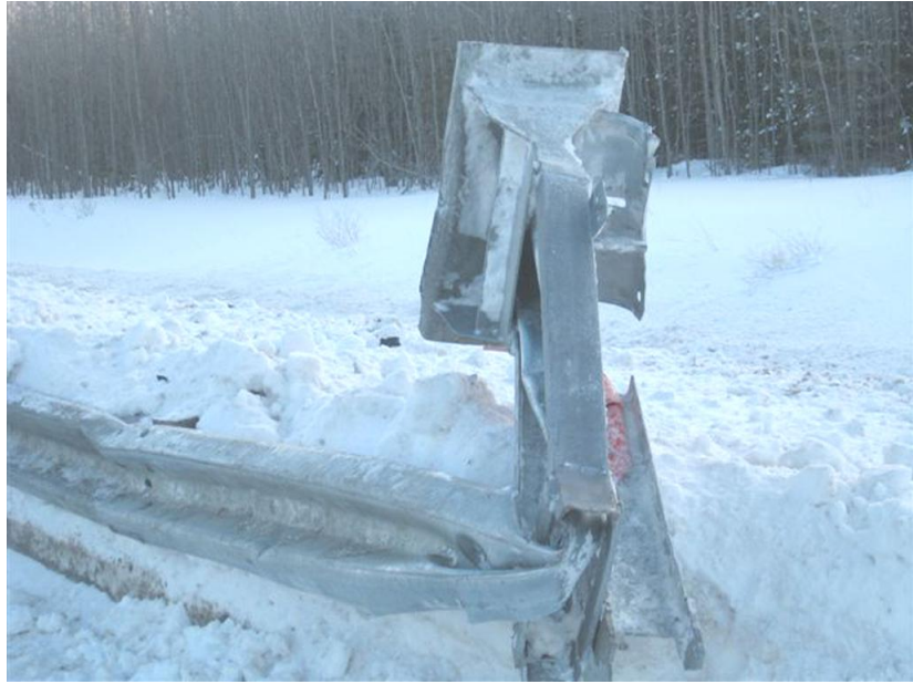
FIGURE 4: Terminal head kinked upward adjacent to snowbank (Source: Brun-Way, 2009)
