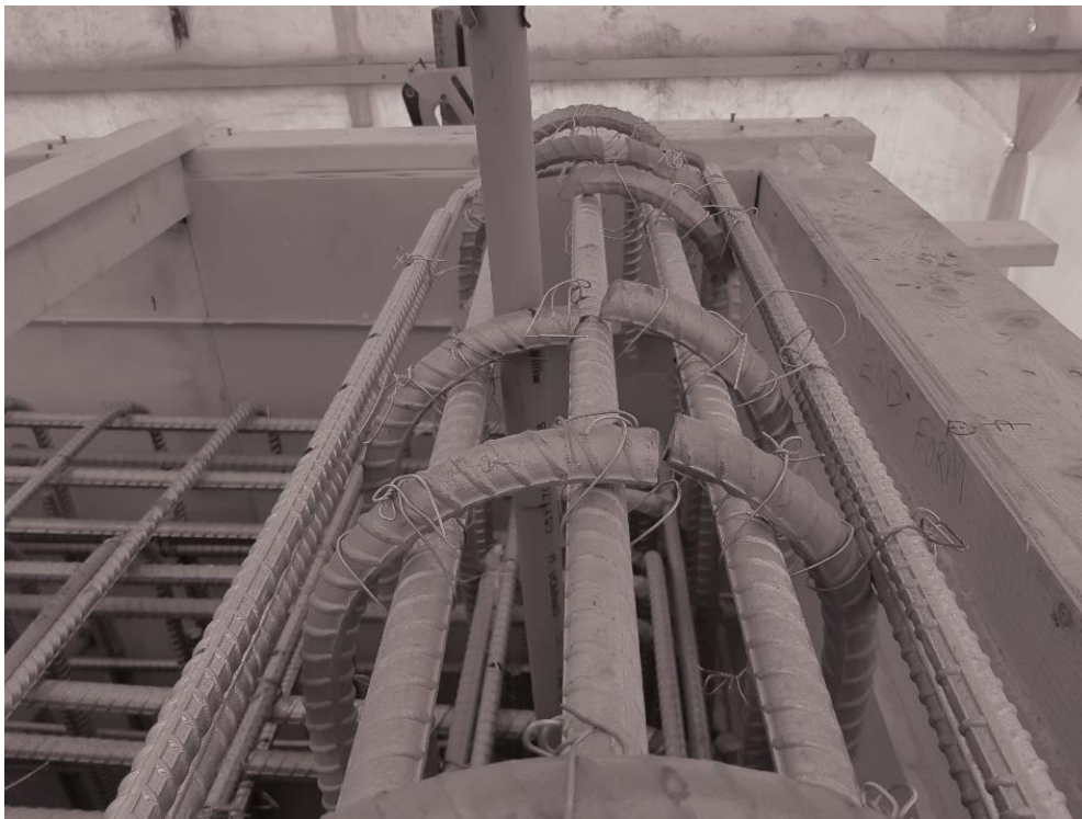
Figure 8: Typical Failure of HDG Rebar (Note bent bars are fractured in two)
