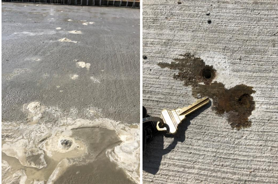
Figure 11: Hydrogen Gas Boils on Concrete Deck Surface Immediately After Pouring (Left); Epoxied Repair of Boils (Right)
