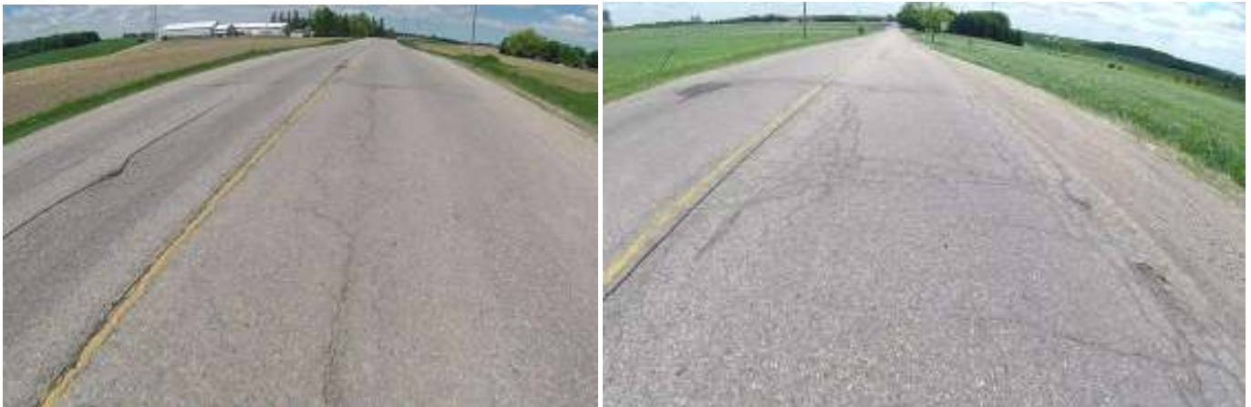
Section 1 – Showing low severity alligator cracking and low severity transverse cracking with good ditches
