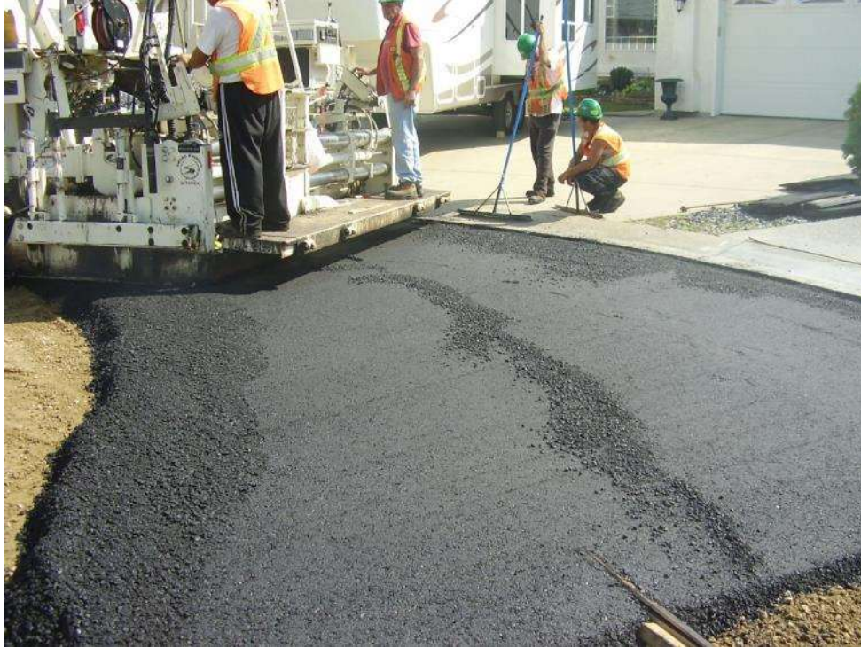
Figure 12 - Placement of the Asphalt on the Granular on 62 Street NW, Edmonton, Alberta
