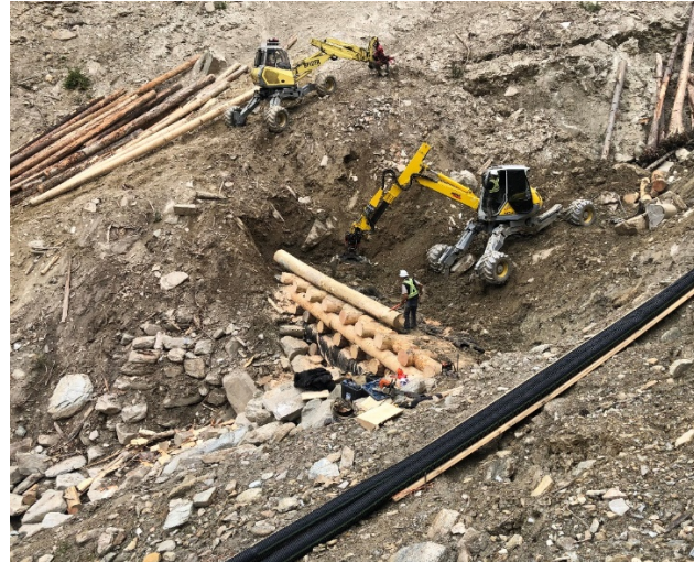
Figure 13 - Log placement for dam construction with spider excavator. Photo by McElhanney (July 25, 2020).
