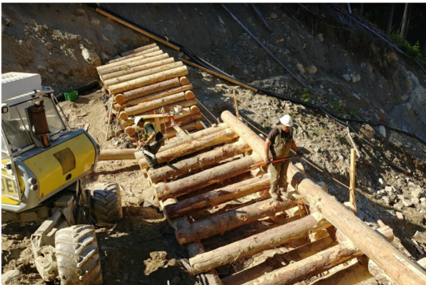
Figure 14 - Final placement and connection of logs completed by hand. Photo by McElhanney (August 18, 2020)
