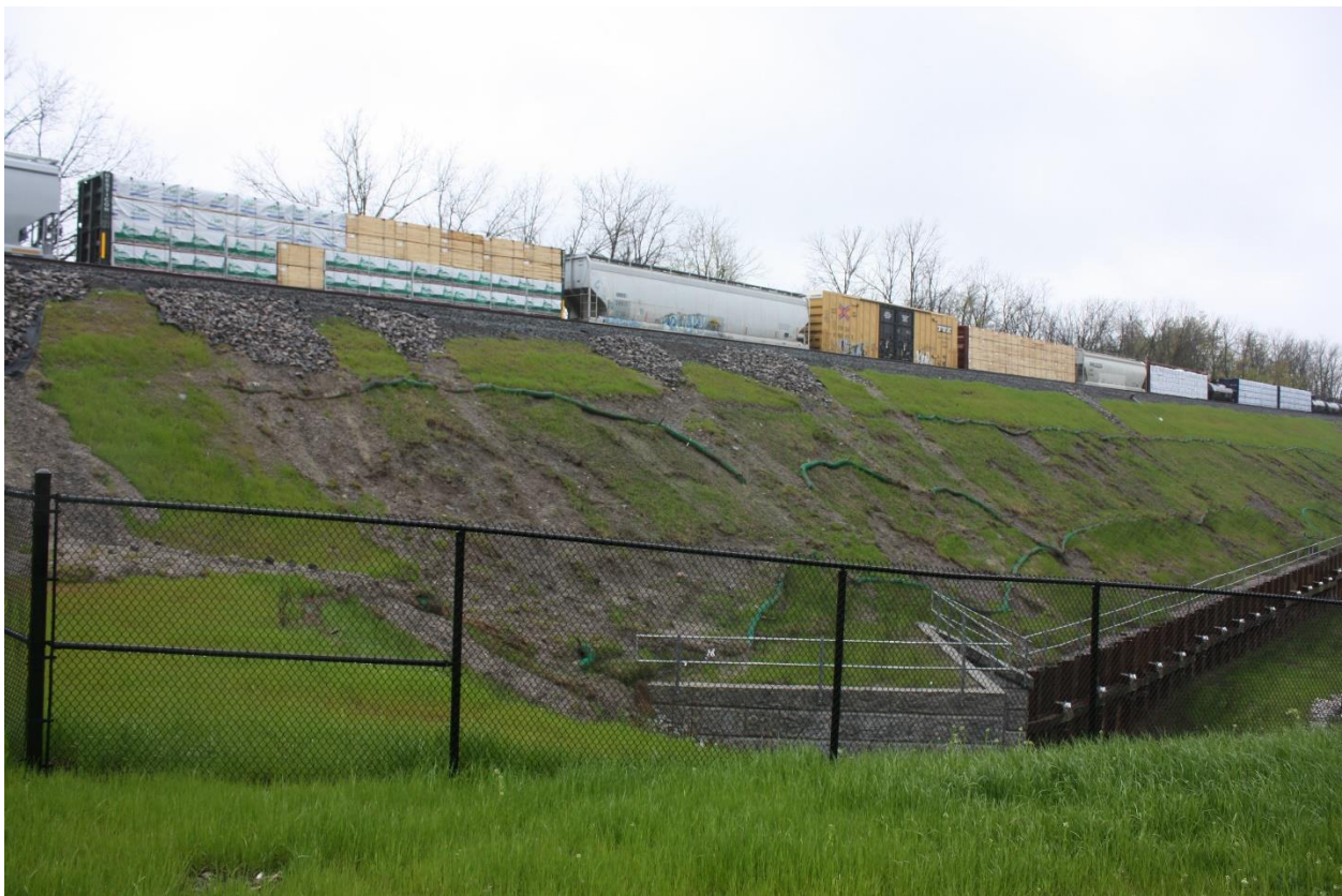
Figure 5. Slope interruption device contributing to surficial soil instability by moisture retention
