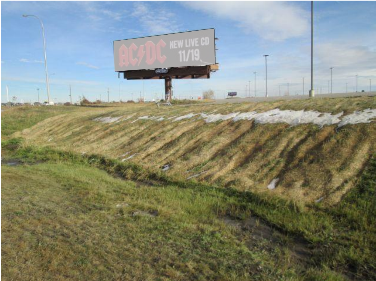
Figure 6. Erosion below Erosion Control Blankets not conformed to soil surface
