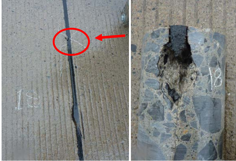
Figure 3: Deterioration Below the Surface of a Visibly Intact Joint on Hwy 417
