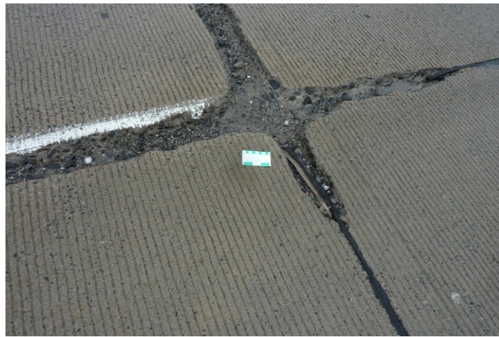
Figure 2: Deteriorated Joints on Highway 417
