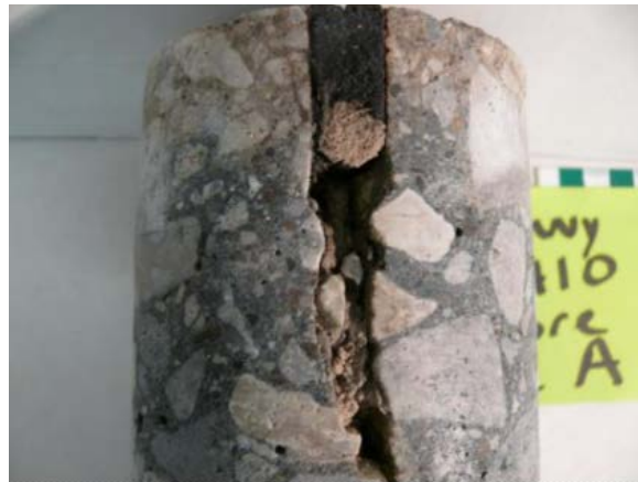
Figure 4: Premature Joint Deterioration (core taken from Highway 410)
