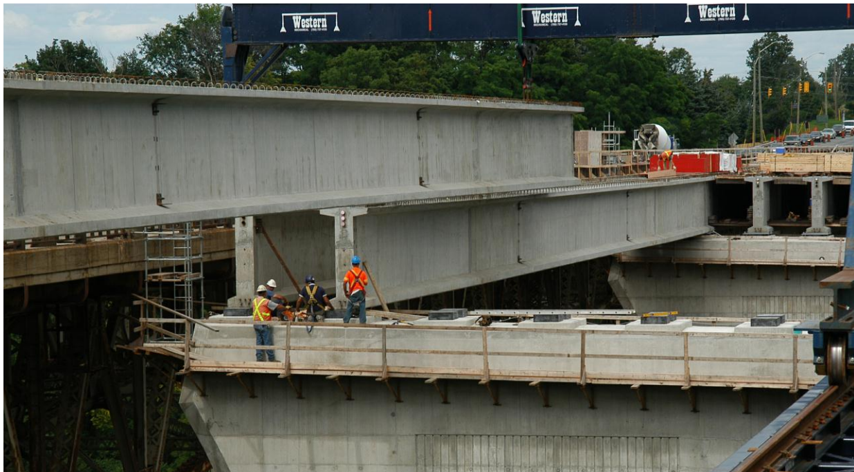
Figure I: Placing 61 metre long, field spliced, precast concrete girders using an overhead gantry
