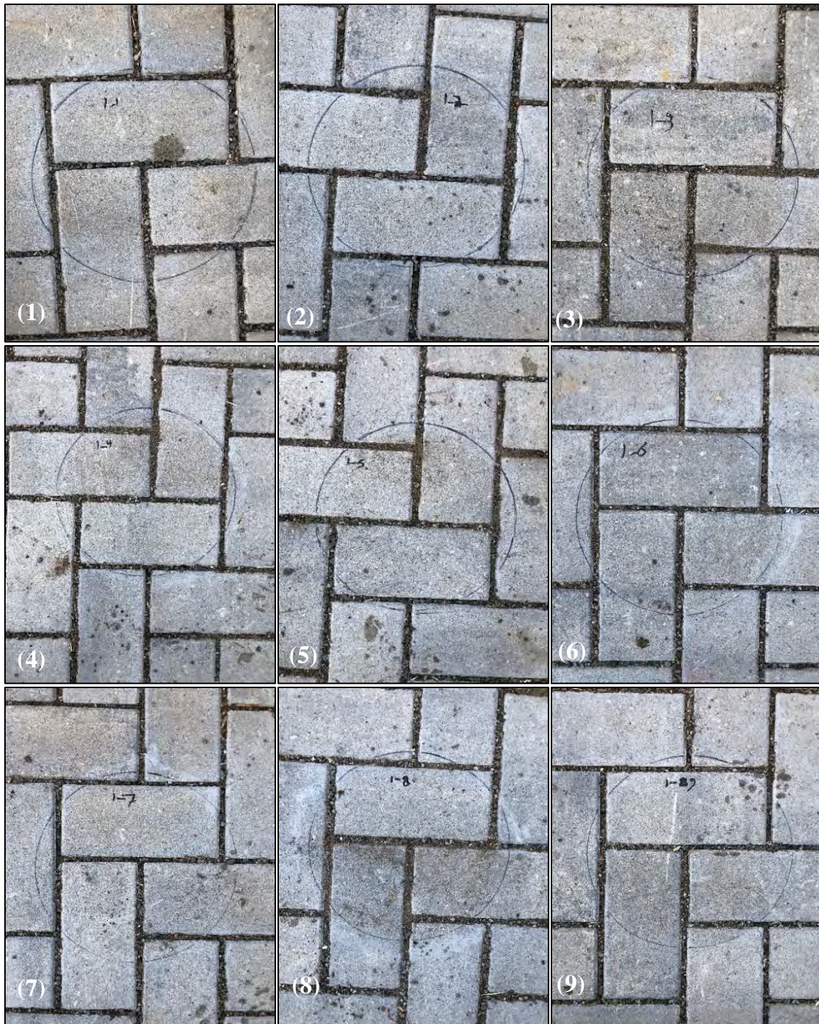
Figure I1: Pre-maintenance photos of infiltration measurement locations (1-9) on Cell 1 (Pave-Tech Typhoon® and Pavevac®).
