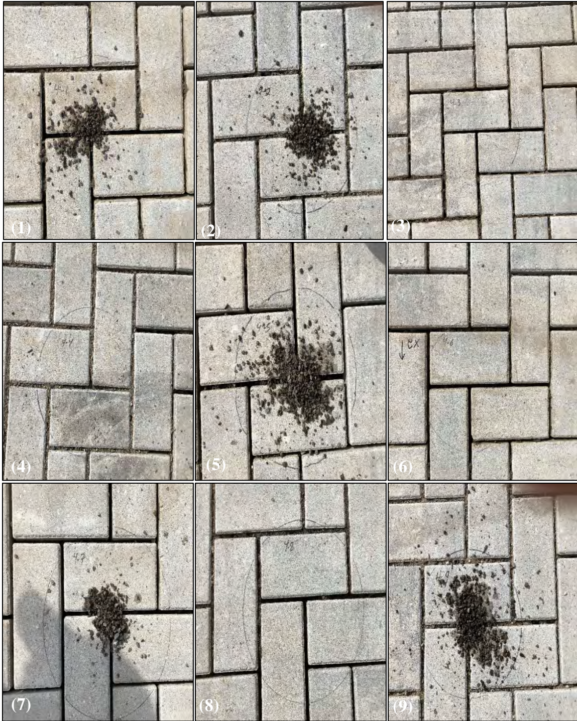
Figure I6. Post-maintenance photos of infiltration measurement locations (1-9) following a vacuum street sweeper on Cell 4 (Elgin Whirlwind).
