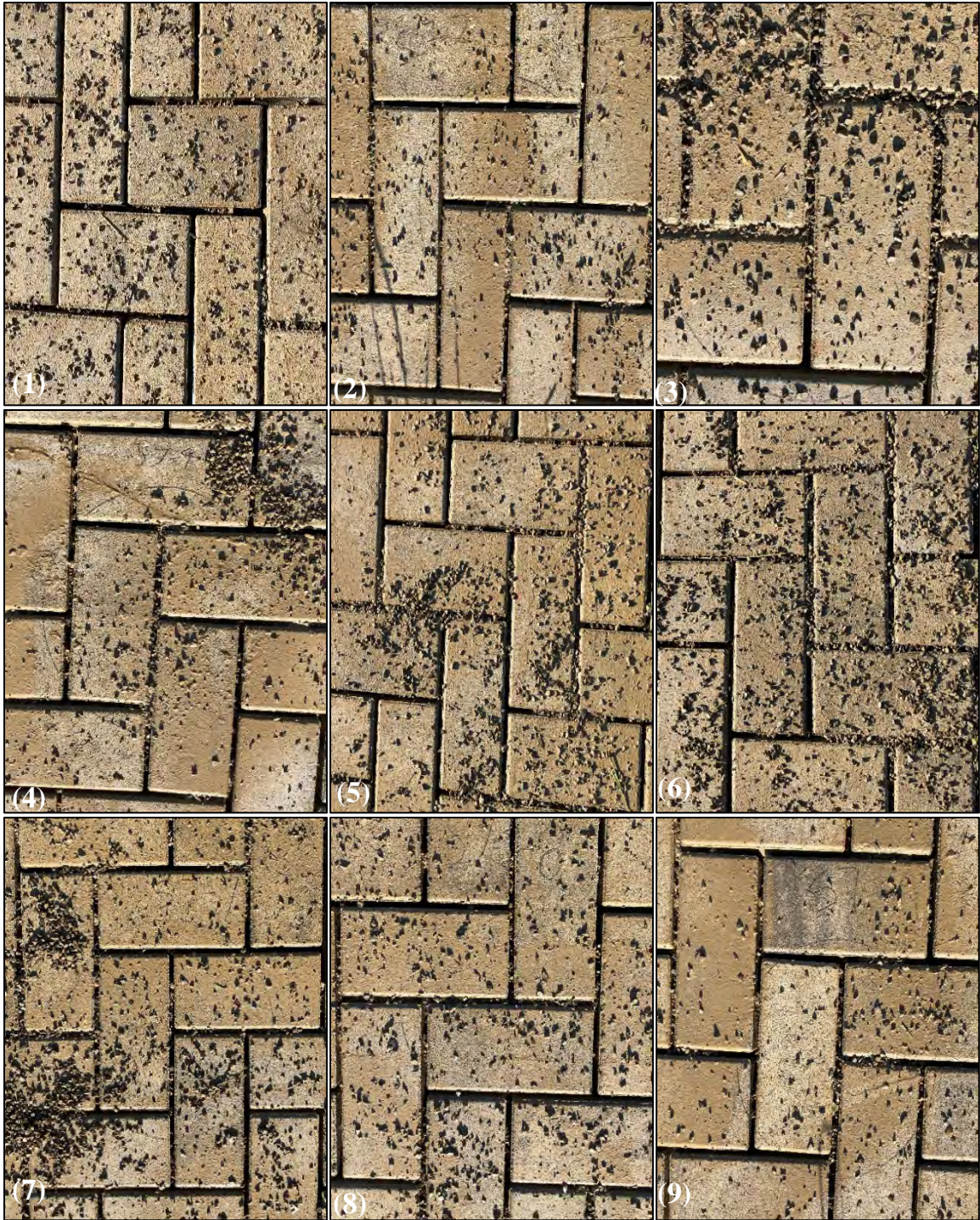
Figure K2. Post-maintenance photos of infiltration measurement locations (1-9) following high pressurized-air system on Cell 7 (Pave-Tech Typhoon®).
