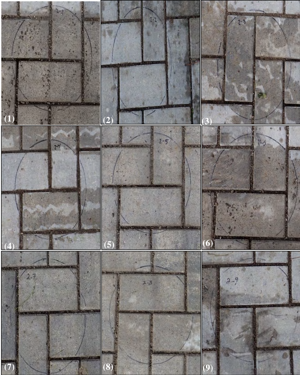
Figure I4. Post-maintenance photos of infiltration measurement locations (1-9) following a regenerative air street sweeper on Cell 2 (TYMCO DST-6®).
