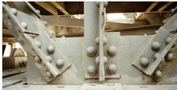
Photo 3. Typical Condition of Caulking of Pack Rust Joints
