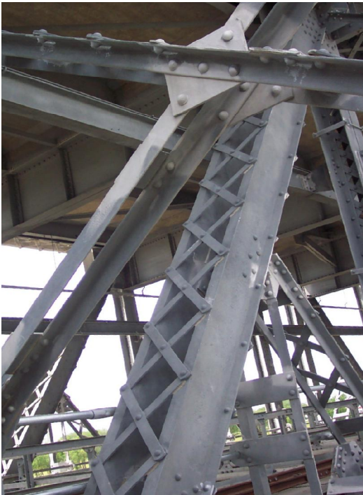
Photo 2. Typical Condition of Coating
